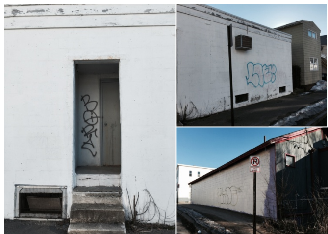
Examples of Graffiti on Existing Buildings
